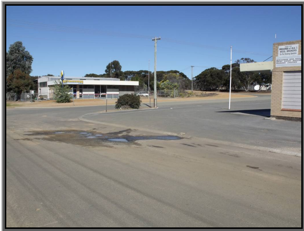
Image 5: Pavement failures on Moorshead Road
